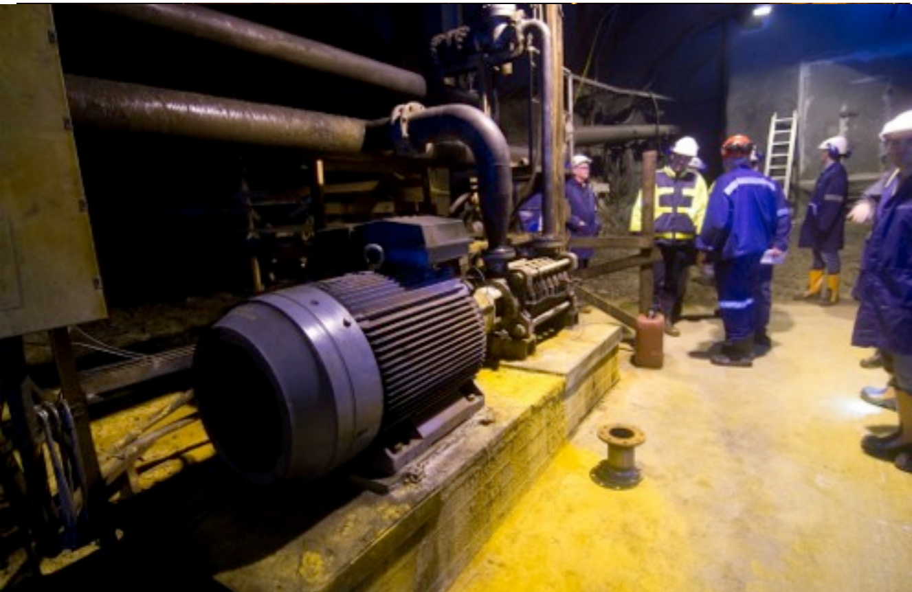
This pump alone takes all the water from 645 m to the surface
